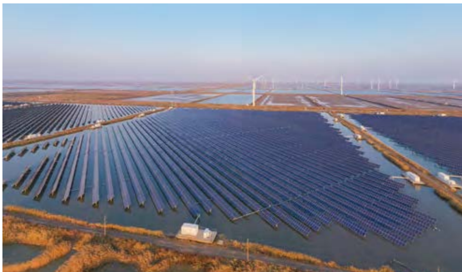
Xiangshui, Jiangsu 120MW solar aquaculture project
