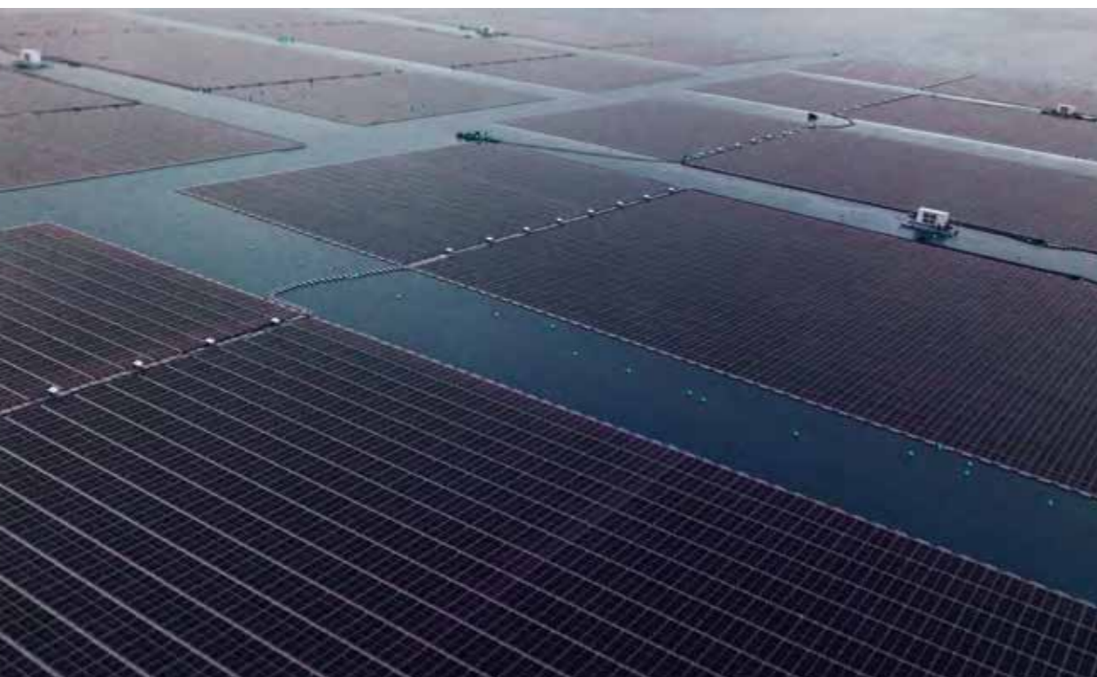
Binh Dinh Province, Vietnam 50.6MW Vertex Dam Tra O floating project
